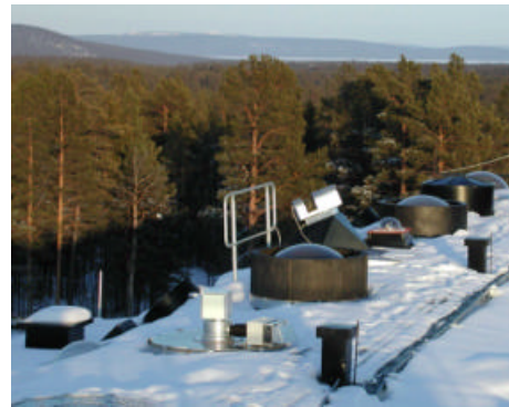
FTIR-solar-tracker on the top of the optical lab in Kiruna, Sweden Operator: FZ Karlsruhe
